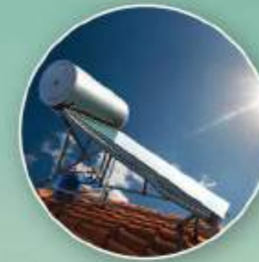
Solar Water Heater
