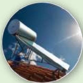
Solar Water Heater
