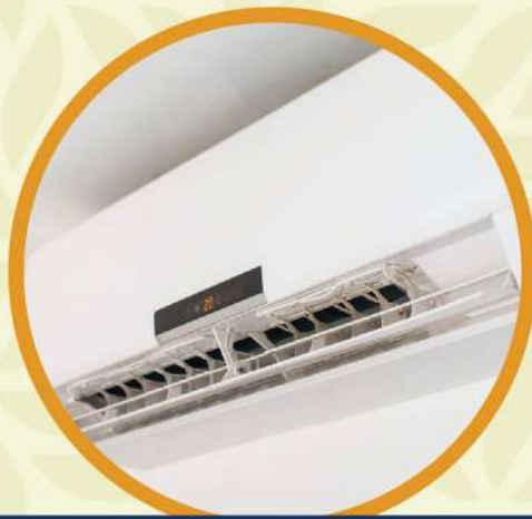
Air Conditioner tiap lantai
